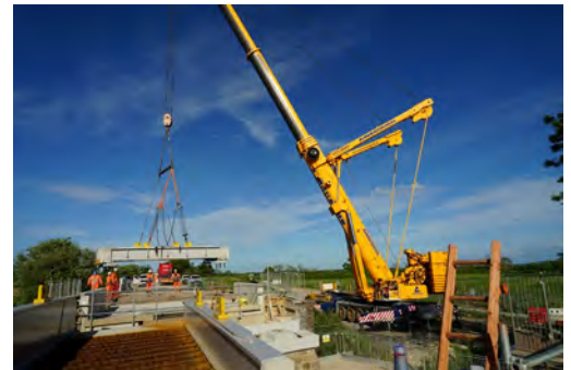
A steel bridge deck is lifted into place on OXD34, Bicester Road, Launton
